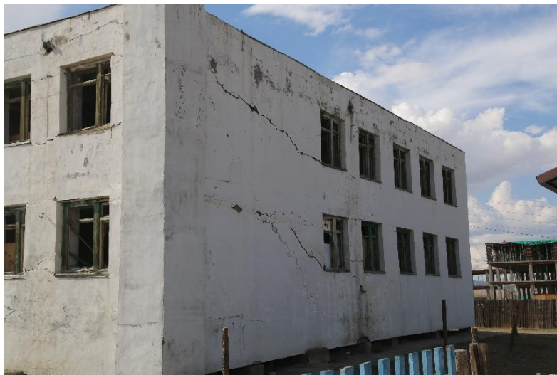
Figure 4.26 School building at Tsakhir soum, Arkhangai province, Crack on the wall due to permafrost thaw
