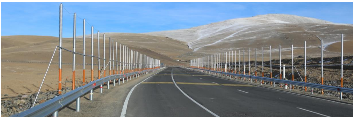
Figure 4.28 Wave on road surface (settlement on surface) in Valley of Chuluut River
