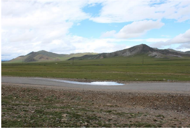
Figure 4.27 Wave on road surface (settlement on surface) in Valley of Chuluut River
