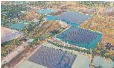
Floating Solar PV, TSB Co., Ltd., Thailand
