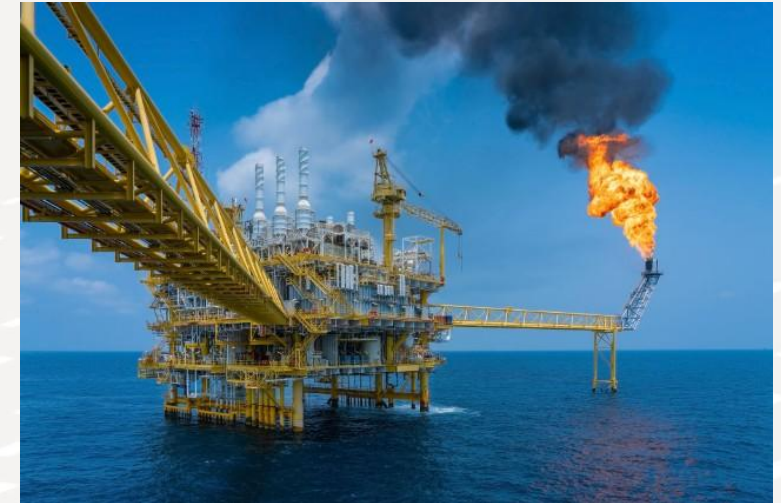
Flaring systems for waste gas
